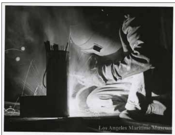
Welder at California Shipbuilding Corporation, Terminal Island from the William A. Bergstrom Collection.
